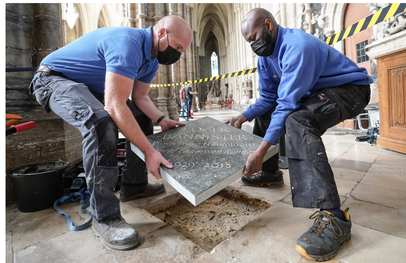
Members of the Clerk of the Works team install the memorial stone to Sir Roger Bannister in the north nave aisle in September.
