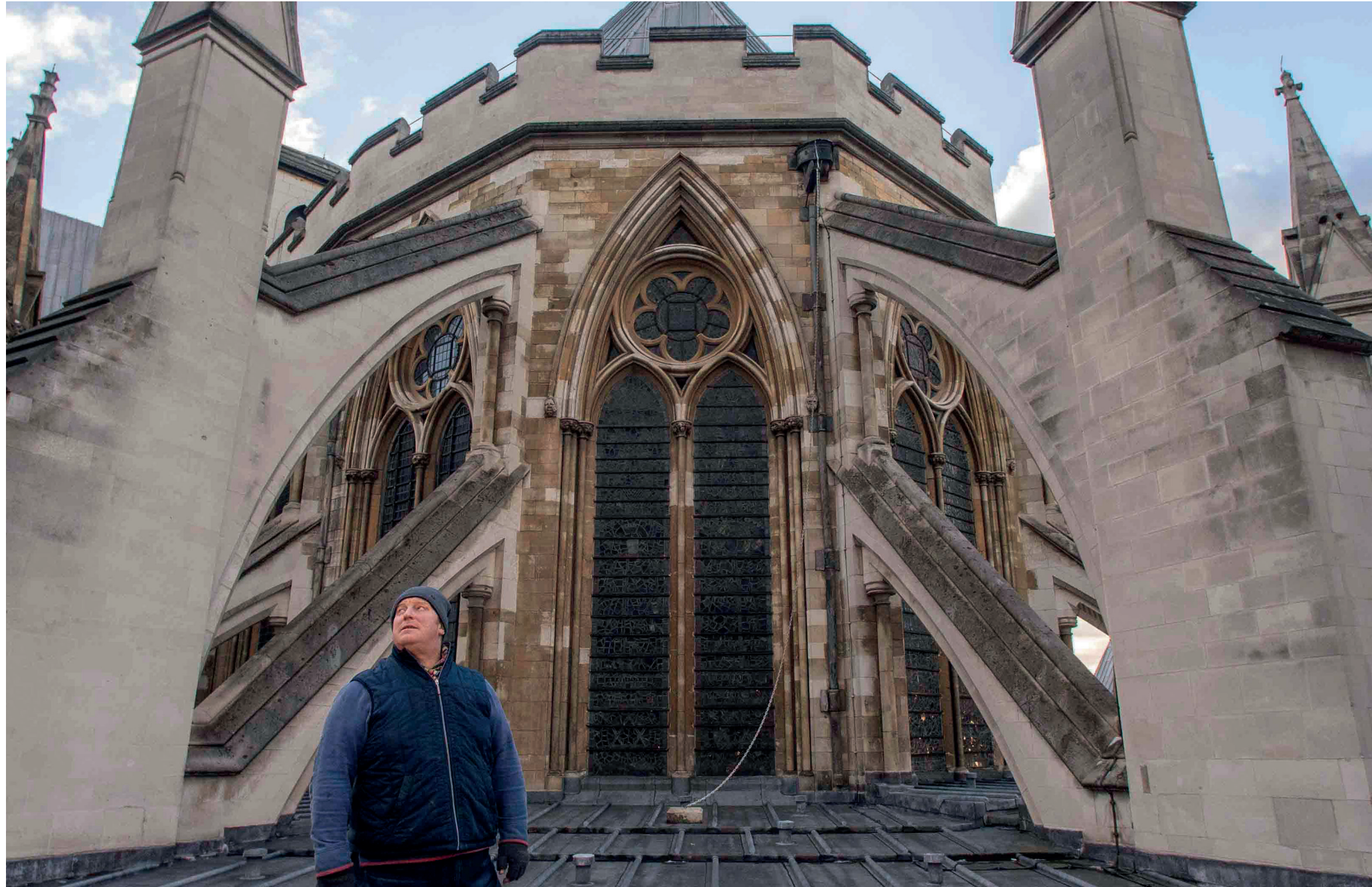
Throughout the Covid-19 closure the Abbey's Clerk of the Works, Ian Bartlett, maintained a regular programme of inspections – including the roofs.
